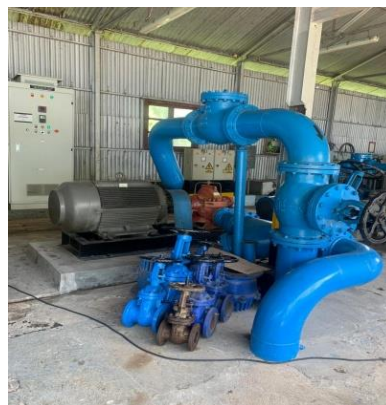
Gambar 2. Pompa Feed Sentrifugal P.100/4
