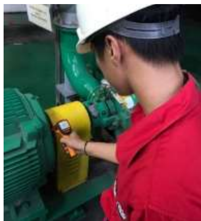
Gambar 6. Check Temperatur Bearing CCWP
