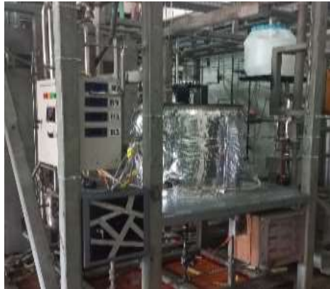
Gambar 1. Fasilitas Heating Control
